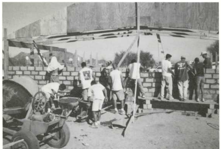
Pepperdine students worked hard over spring break 1999 helping with Project Serve San Felipe. Here, students meet the needs of one family by building them a home.
